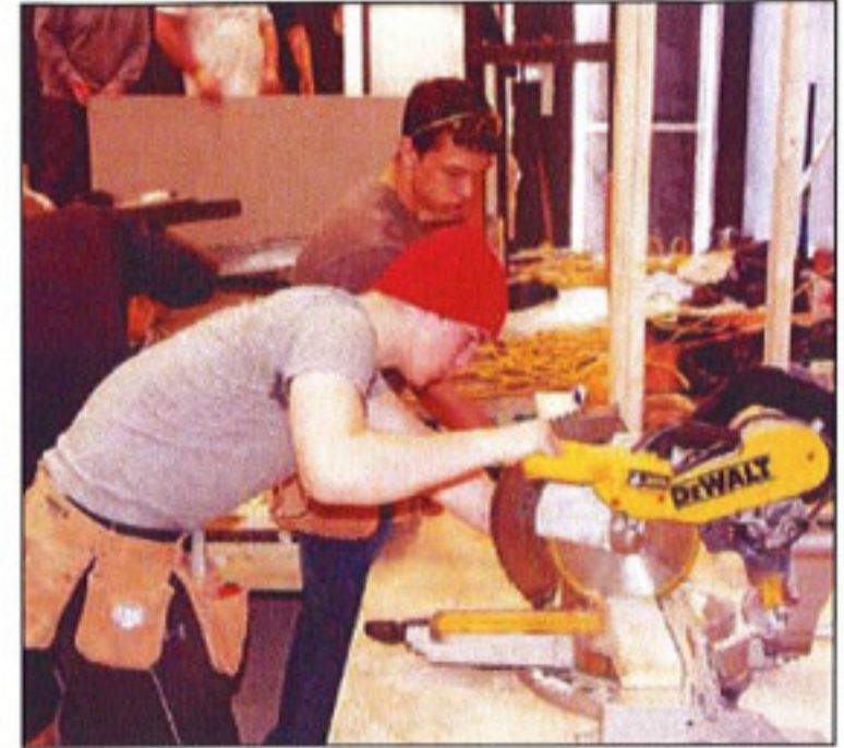
Cardinal Carter student Luc Ribble cuts a length of two-by-four while fellow student Mack Butler looks on as part of a project to modify and extend the stage at The Bank Theatre Wednesday, Feb. 17. A group of 14 from the school, made up of High Skills Major Construction program students and others interested in signing up for the course, conducted the project.
